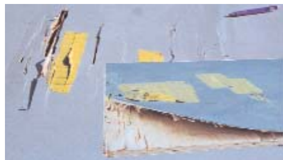
Floor problem with poly-deck
