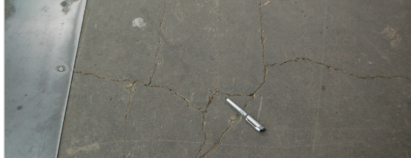
Prior to ResinDek repair, steel plates had to be attached on top of the concrete mezzanine floor so pallet truck wheels could continue to roll.
