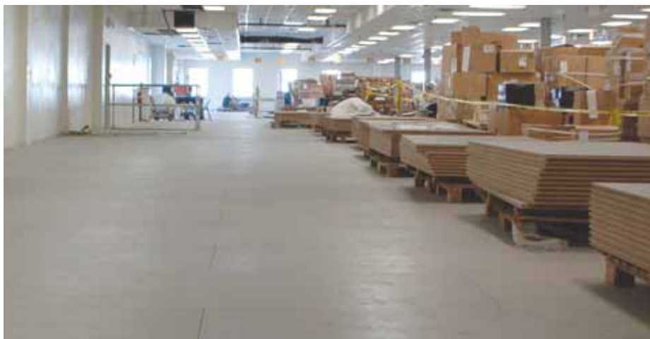
ResinDek installed and loads moving easily
